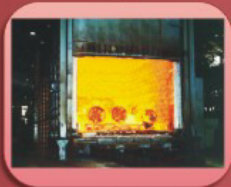
- Pit Type Furnace -
